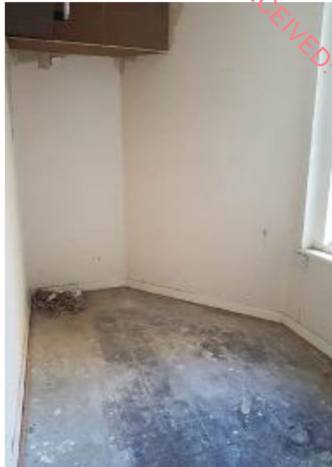
Plate 138: Small room with partitioned wall showing signs of water damage
