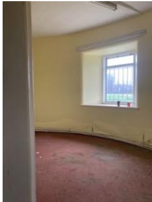
Plate 309: Lower ground floor, within rounded bay. Evidence of water ingress at base of walls.
