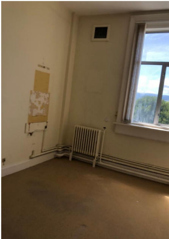
Plate 174: 2 nd floor level typical study room to front (east) on first floor with signs of water damage
