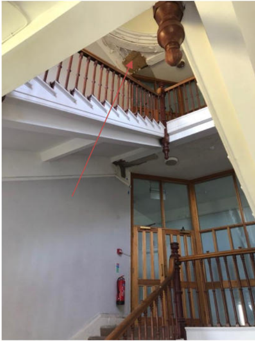
Plate 191: Damage to ceiling above main stairwell.
