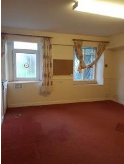
Plate 133: Dormitory at lower ground floor level. Note water ingress
