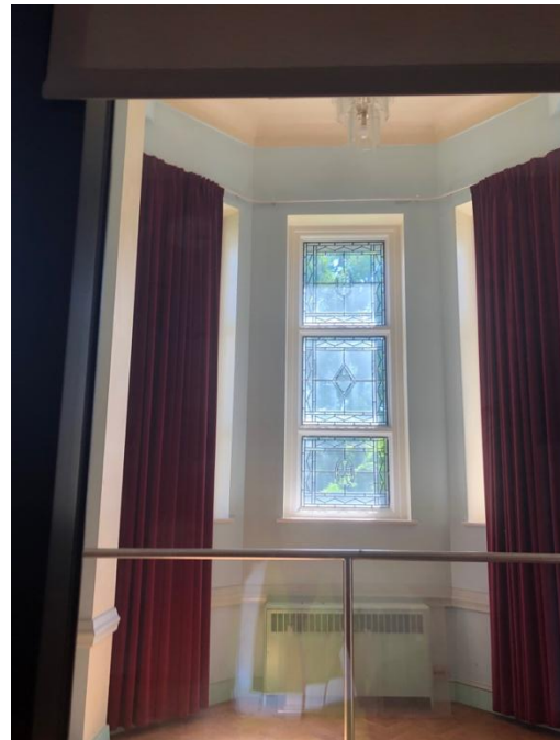
Plate 320: Leaded windows in southern gable. Note water ingress at ceiling level
