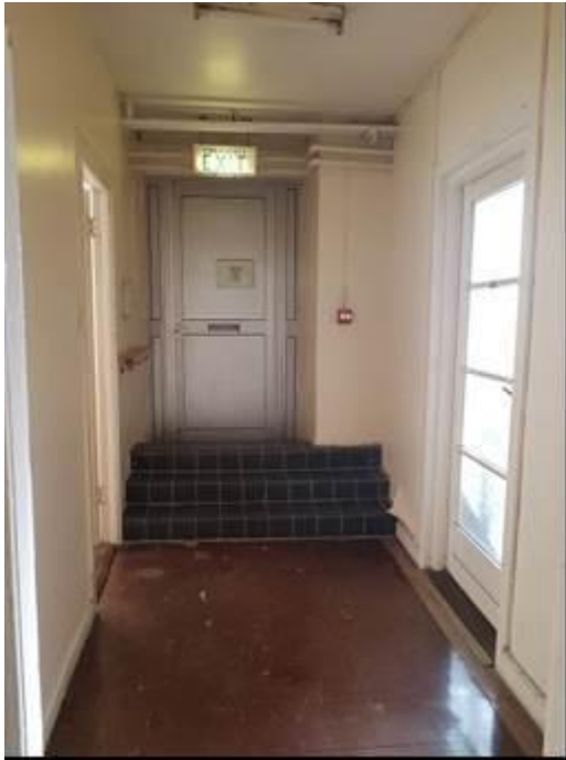
Plate 341: Fire door within central corridor with flood relief barrier evident
