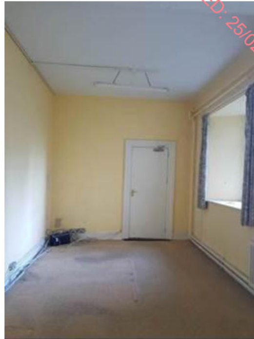
Plate 299: Evidence of water ingress at base of wall.
